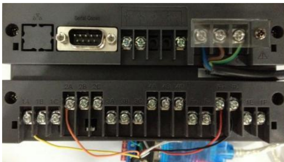
Fig. 10 Cable connection between instrument terminal and HWR330B
